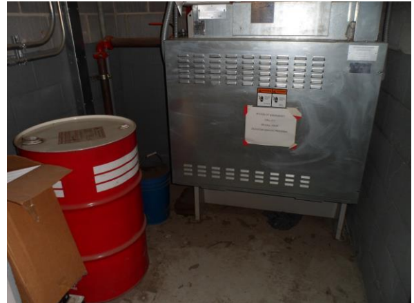
Photo #14 View of elevator hydraulic room and 55-gallon hydraulic fluid drum
