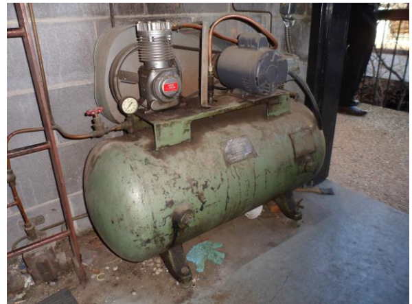
Photo #28 View of air compressor no longer used in mechanical room on second floor
