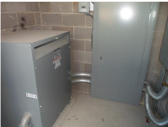
Photo #29 View of pad mounted transformer on second floor
