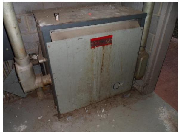
Photo #18 View of pad mounted transformer in electrical room
