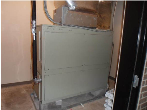
Photo #19 Typical view of HVAC system
