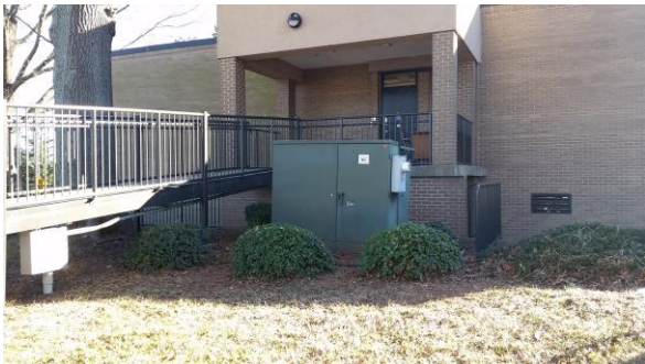
Photo #11 View of pad mounted transformer to the west of site building
